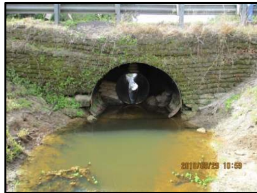
Picture 1: 36" CPEP in 103"x71" arch pipe
